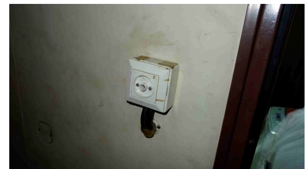
picture 25: damaged light switch
