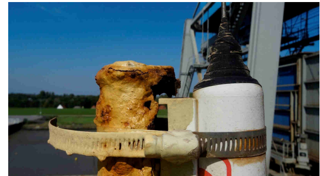
picture 11: rusted foundations
