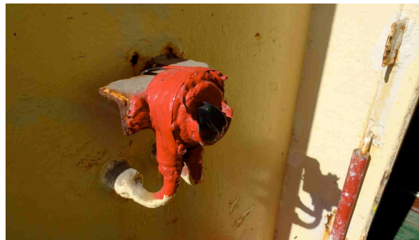
picture 9: switch, repaired by tape and some cable
