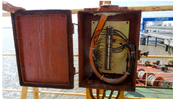
picture 7: unsafe electric installations
