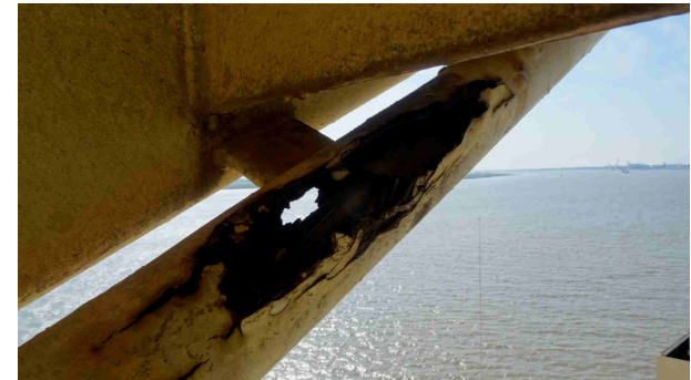
picture 10: rusted pipes
