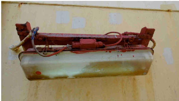
picture 4: damaged emergency light
