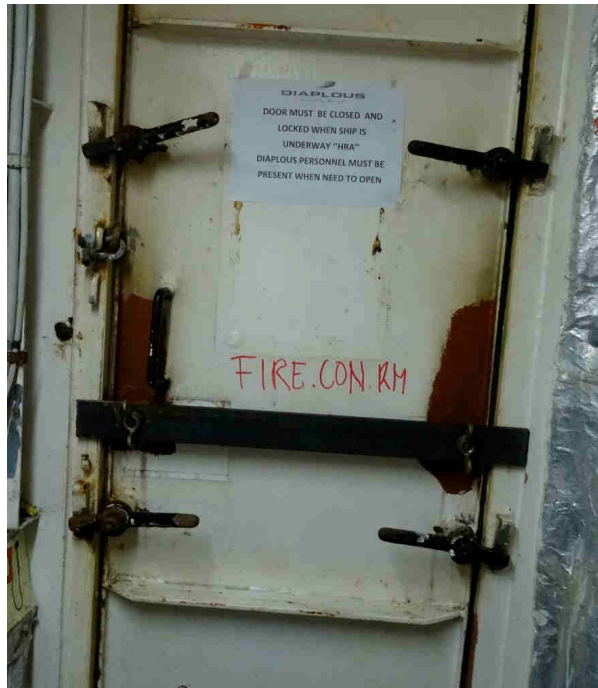
picture 33: Entrance to fire station secured from inside, so in case of fire not possible to reach equipment
